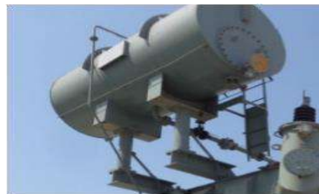
Fig:- Conservator Tank
